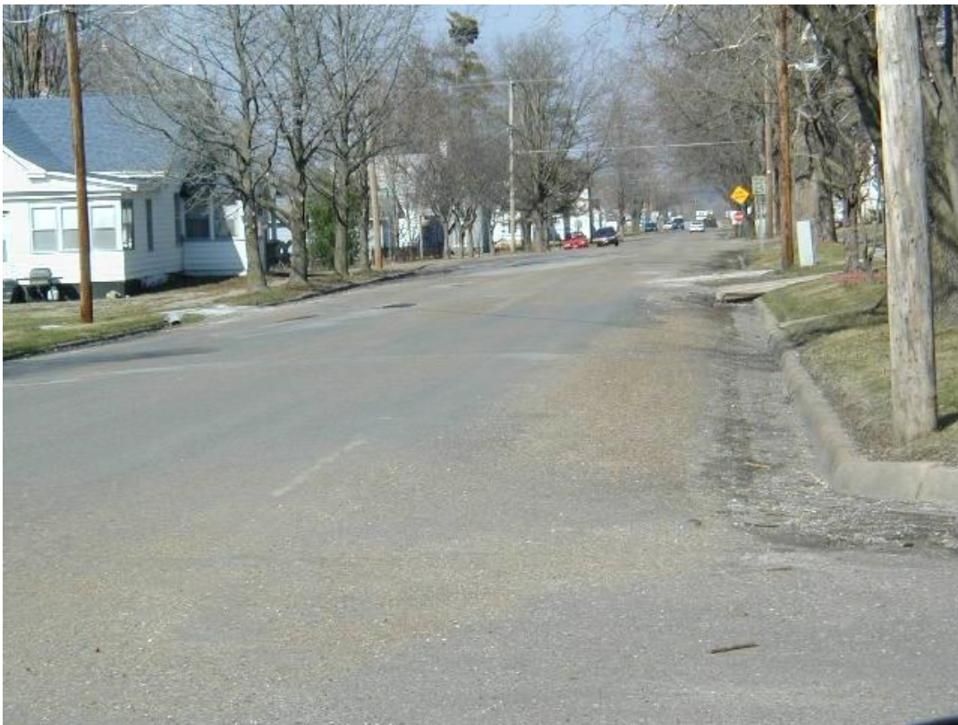
Road still needs to be swept to remove debris.
