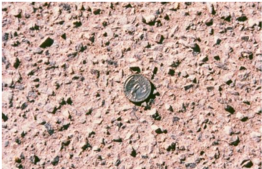
After sweeping – notice the loss of the larger aggregate.
