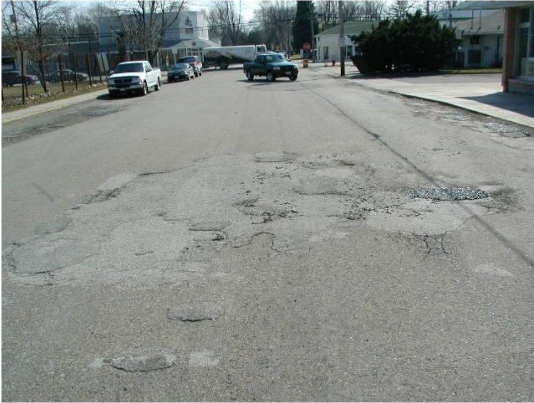
Patch on patch on patch, there may be underlying causes in the base.
