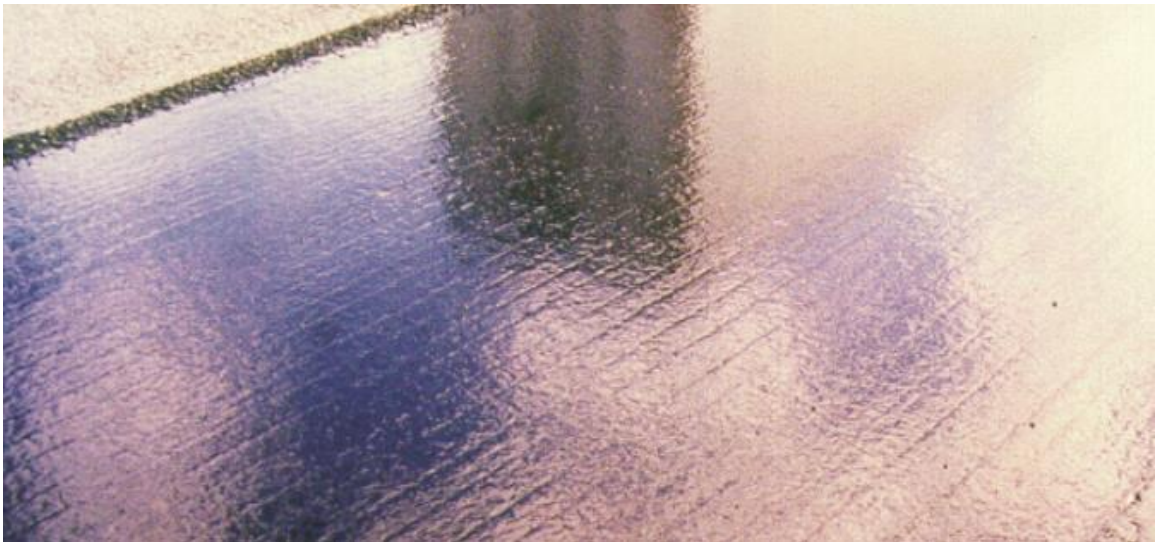
Example of streaking caused by incorrect spray bar height (notice streaks).
