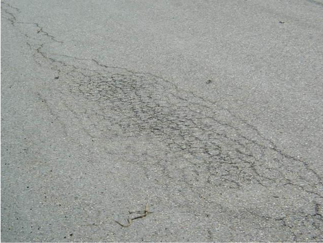
Isolated alligator cracking with minor cracking.
