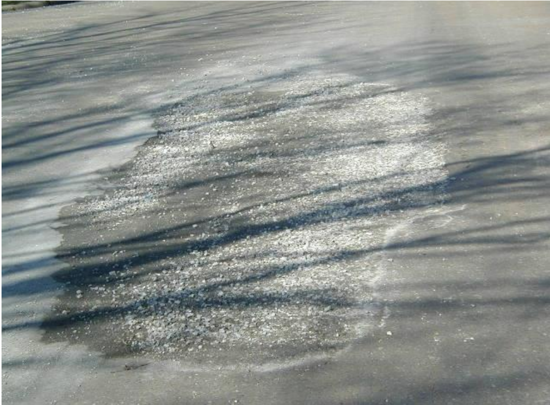
This is an aggregate patch, if it was placed on top of the existing bituminous, it will most likely fail.
