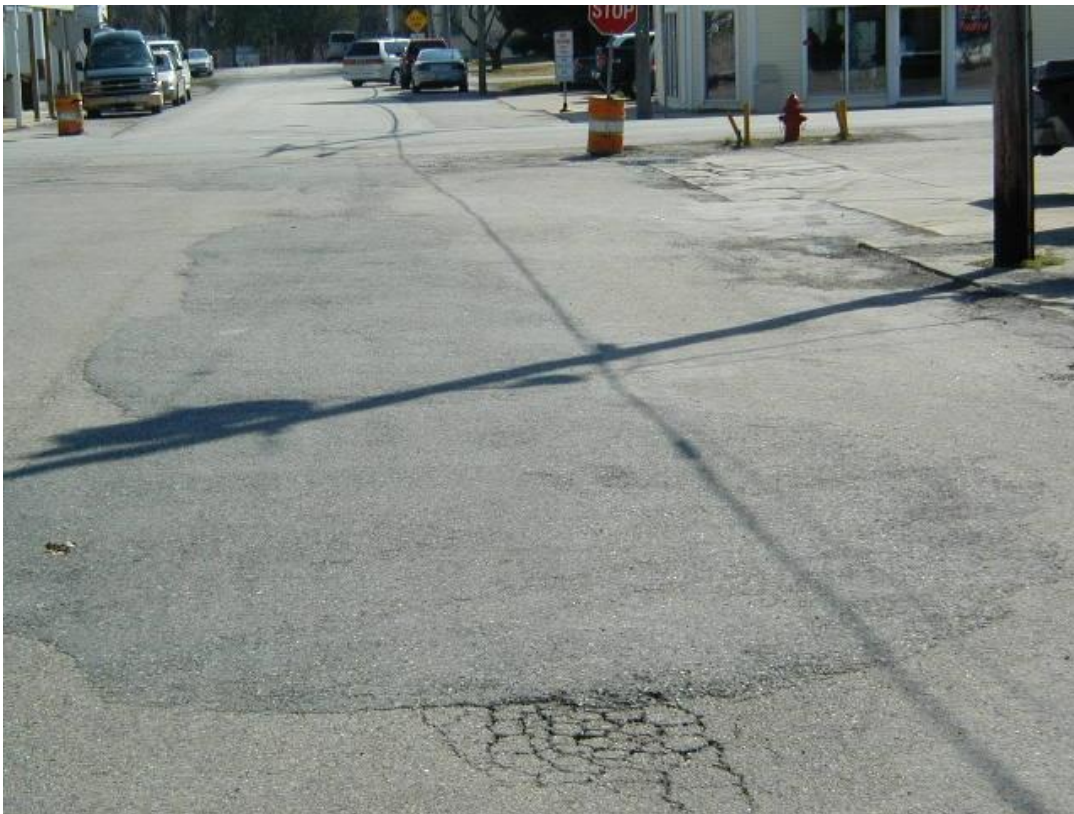
This appears to be good patch, but should have been extended.
