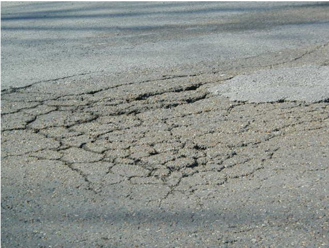
Isolated alligator cracking with major cracking.
