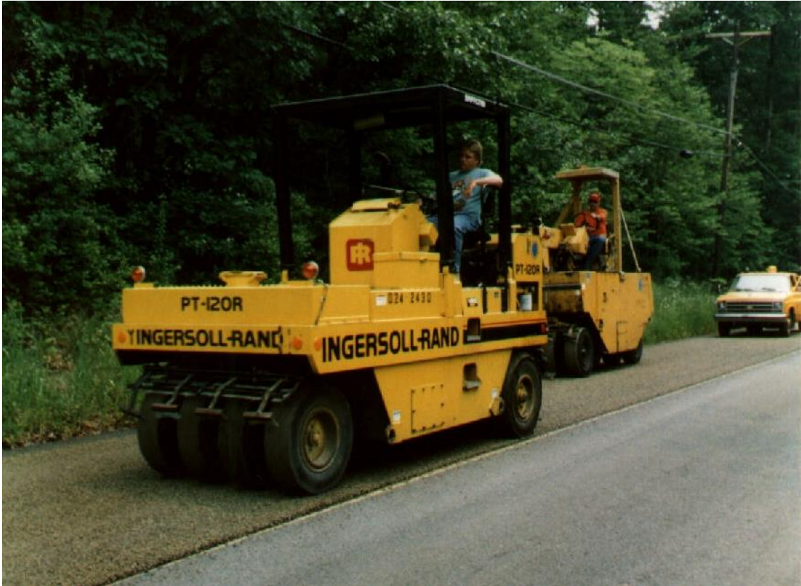
The use of pneumatic tire rollers is required. Steel rollers will crush the aggregate.
