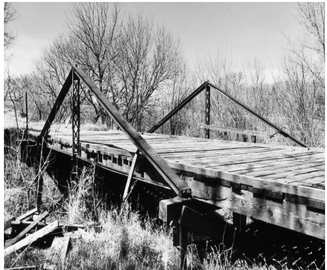
A contract for a bridge inspection should be executed about six months before bridge inspections are due. Above is a 1910 Kingpost truss bridge in Republic County.
