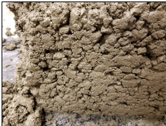
Figure 26. 30.4 fl oz/yd 3 : Too many surface voids.
